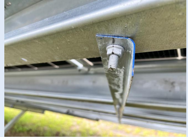
Angle Bracing on Fixed-tilt PV Frame
