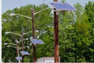
Up to 40 MW of pole-attached neighborhood solar
